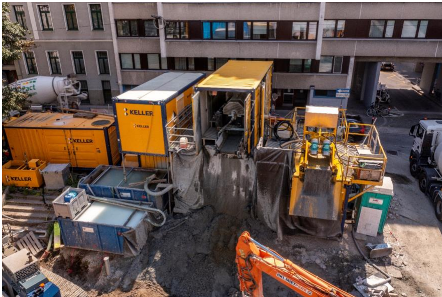
Fig. 4. Site installation at site "Z", from right to left: storage tank with shale shaker, decanter (open doors) over slurry conditioning. The blue basins are used for final pH regulation
