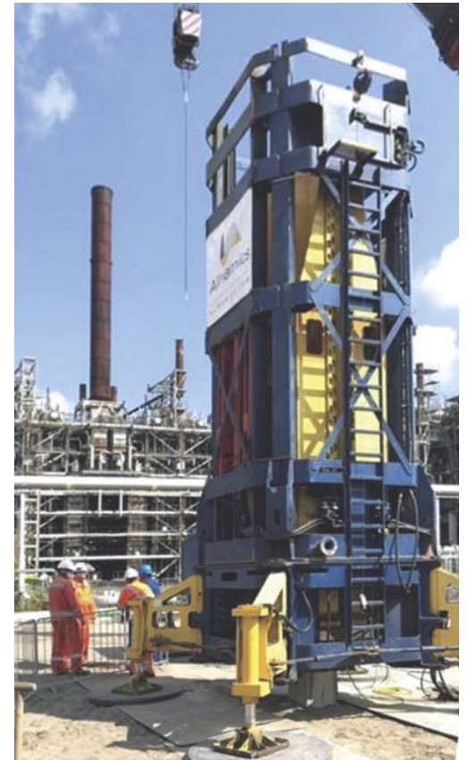
Figure 2 – Pile load tests, like the StatRapid test, can help to eliminate uncertainties in pile performance.
