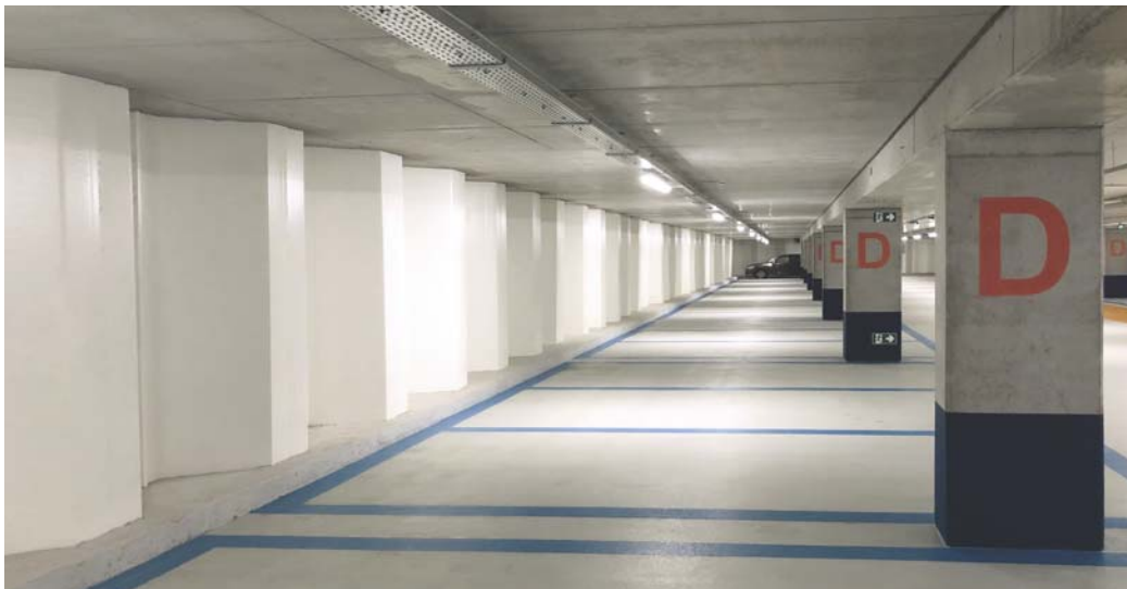
Figure 1 – Permanent steel sheet pile wall of an UCP – Parking Miroir, Brussels, Belgium.
